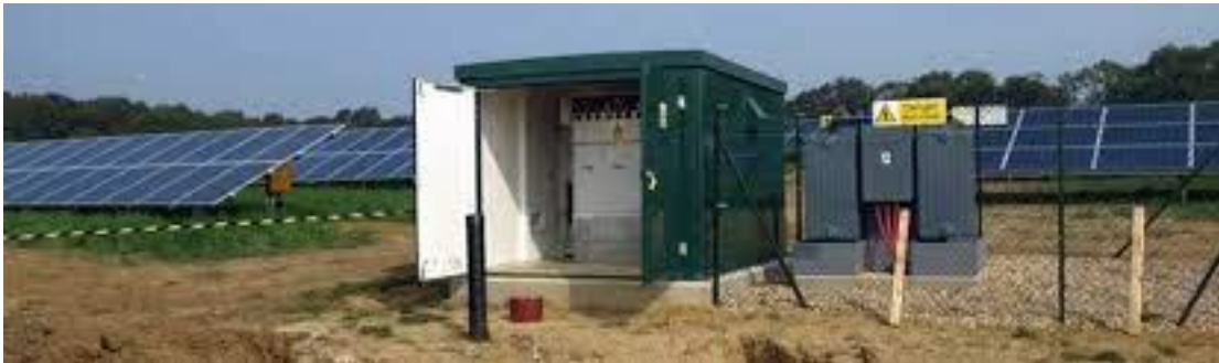
Photo 31: On-Site Supporting Equipment (example only)
